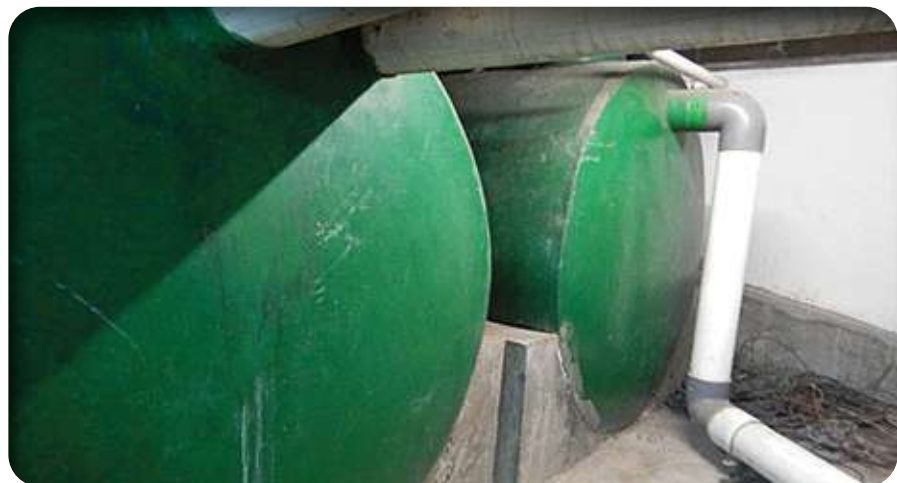
Tempat pengolahan air limbah | Waste water treatment plant
